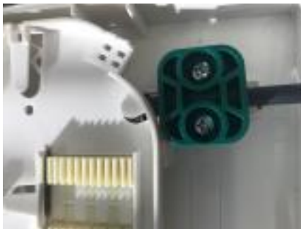
Cable Clamp in JW2 Box
